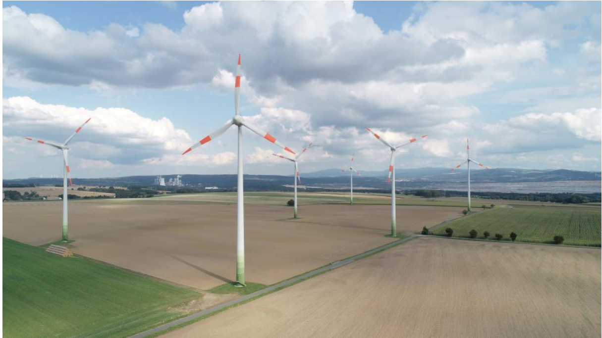
Photo: Part of the existing wind farm in Mittelherwigsdorf
